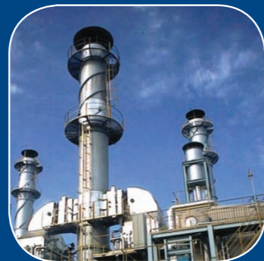
Romelectro, Romenergo, SAEM, Tecnoservice, Termoelectrică, Transelectrica, Water management companies a.s.o.
