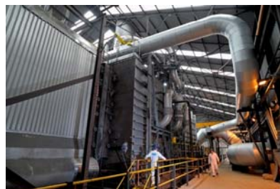
Doosan Babcock OxyCoal Clean Combustion Test Facility. Image courtesy of Doosan Babcock
